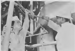
Bruno Thode, a metal tradesman-Pipe, (at right) and Venancio Solognier, building tradesman-Carpenter, install new fog nozzles on the PCAR fire water line system.
